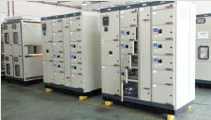
M-Cube Fixed Type Switchgear
